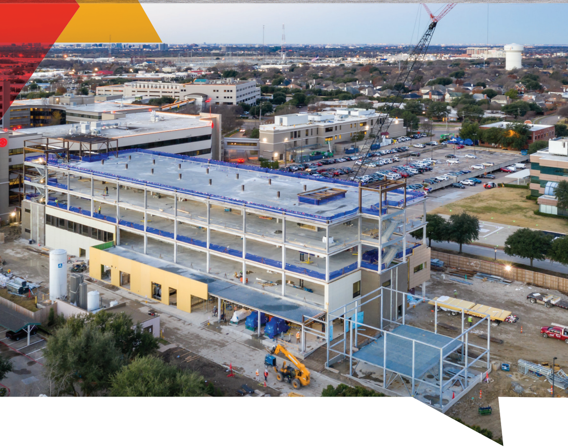
Work on the HCA Medical Center in Plano, Texas, by the Brandt Companies is scheduled to be completed in the third quarter of 2019.
