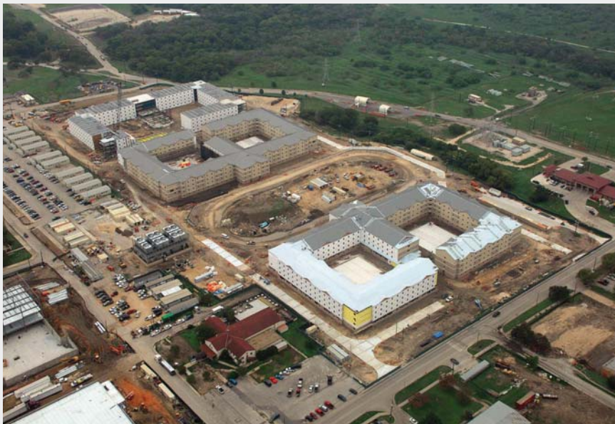
At the center of each facility's footprint, site-built construction. Once the site-built portion is completed, the modular components are added, extending out as residential wings in the building. At each of the corners, site-built construction is used to create mechanical rooms and stairwells.
