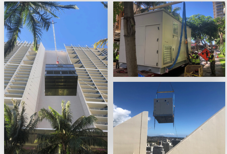
Left: A cooling tower is lifted on the roof Right: A PCP is rigged to be lifted on the roof
